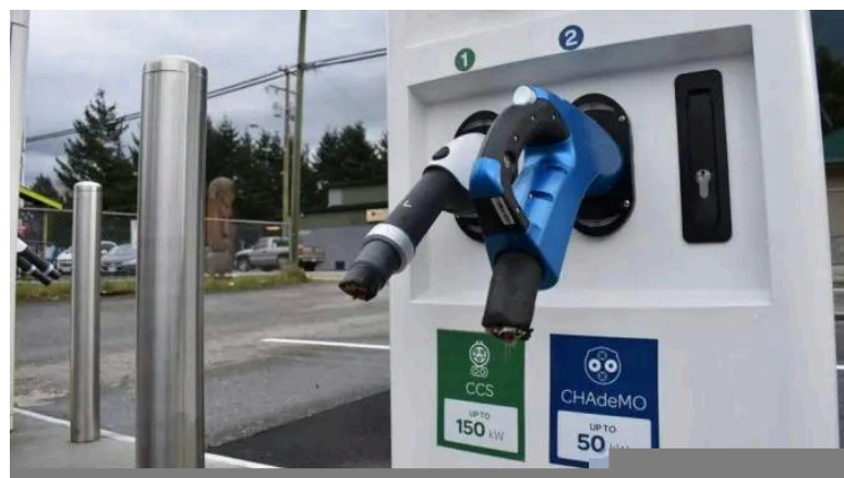
Electric vehicle charging station with severed cables.
