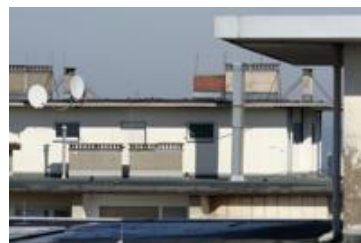
Power cable on the roof
