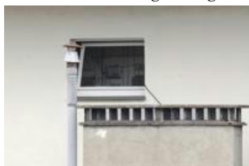
Power cable reaching the socket
