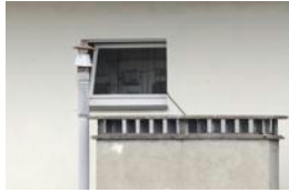
Power cable reaching the socket
