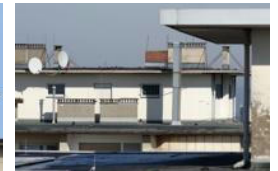
Power cable on the roof
