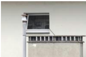
Power cable reaching the socket
